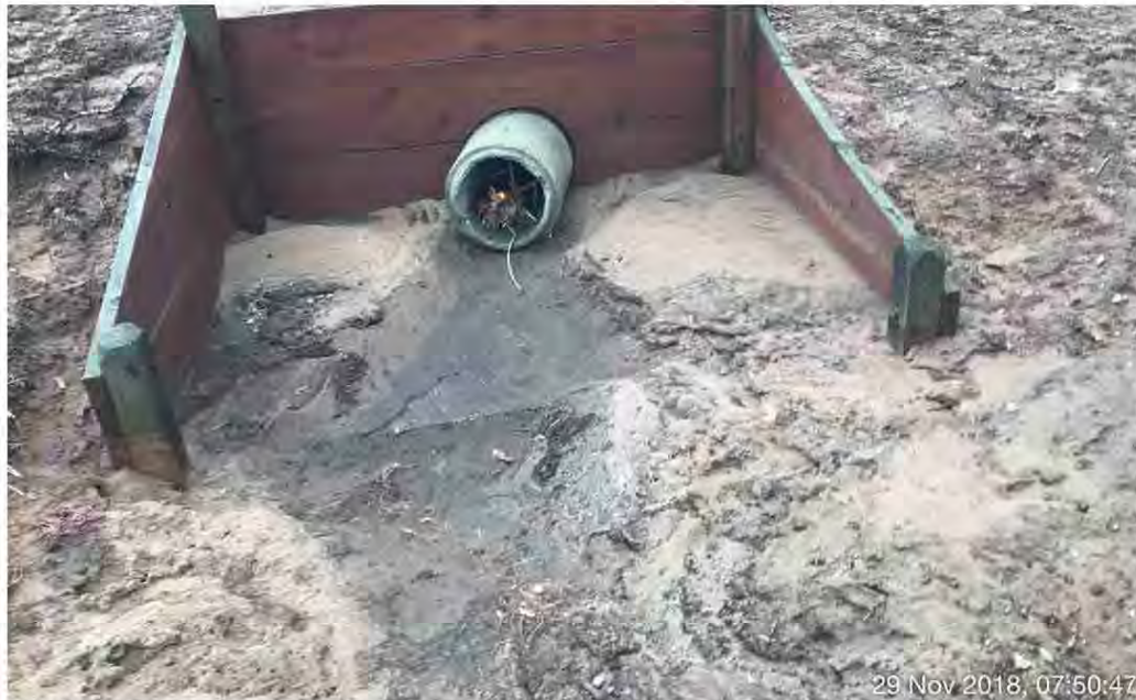
Photo 8. Scour at pond inlet pipe, 11/29/18
